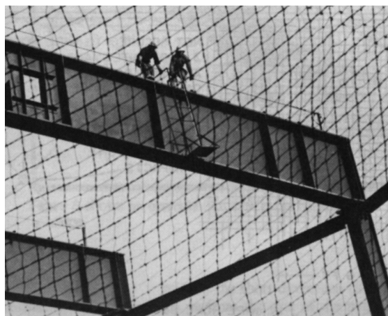
Figure 1. A typical safety net installed under steel workers who are securing a roof beam.
